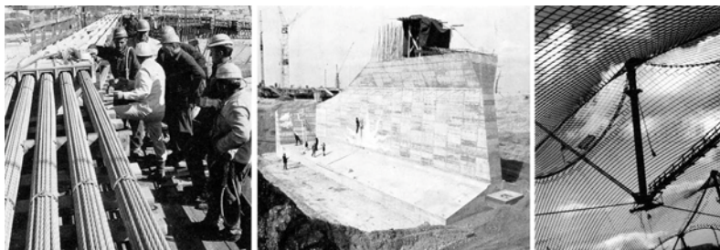
Fig 38: Ten bundles of 55 strands for the main edge cable. Fig.39: Heavy weight foundation for a lightweight structure. Fig.40: Flying mast, an invention of Frei Otto and his team.
