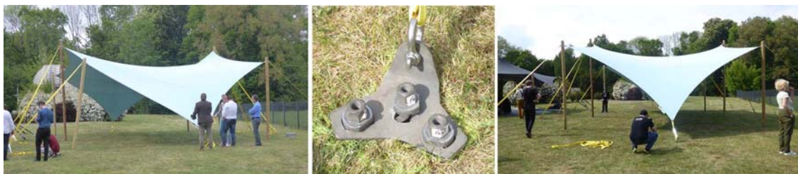
Fig.143: an anchor loosened. Fig.144: reinforced anchor. Fig.145: the result was satisfactory
