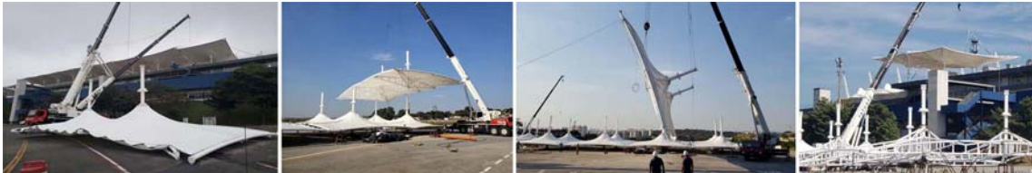
Figs.63,64,65,66: Formula 1 Interlagos Pavilion 2. Lack of accessibility and space forced to assemble the modules outside and install them with cranes.
