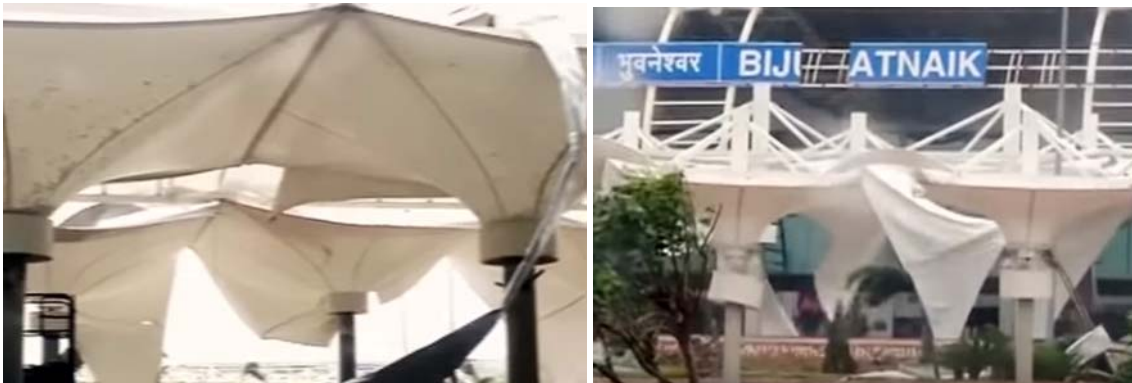
Fani cyclone damages - May 2019: Bhubaneswar International Airport
