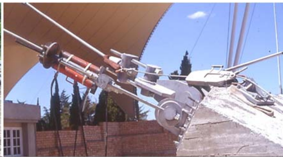
Auxiliary plates, bores and anchors could have been integrated in the design.
