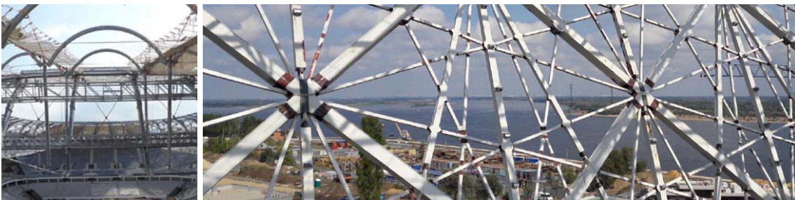
Installation of the Volgograd textile roof (left) and steel framework of the façade (right)
