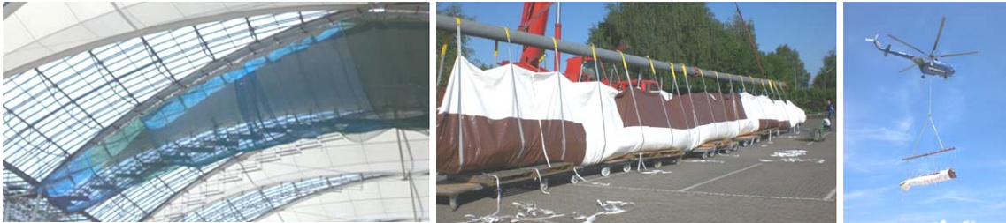
Munich Airport Center. PTFE-coated glass-fibre fabric. 5 of 7 existing panels were replaced while the airport was in full service.
