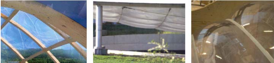
Foil cushions with supporting structure, cable net and belts
