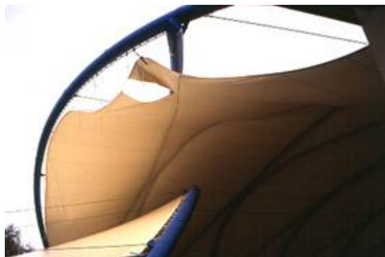
Poor maintenance. Jaén, 2002
